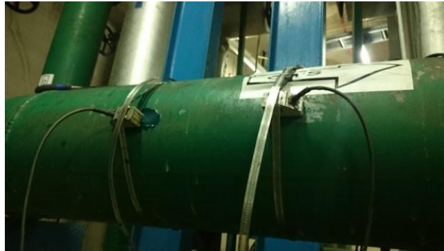
Figure 4. Flow meter Ultrasonic (Transmitter and Receiver)placed on the Pipe
