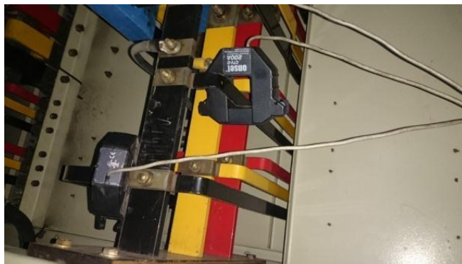
Figure 5. Power meter (Black with Wire) is Clamped onElectricity Panel
