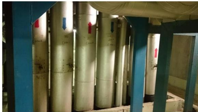
Figure 2. Chilled Water Pipe (Supply and Return)
